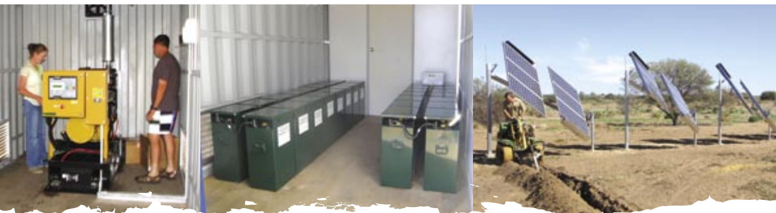
Clockwise from top: Arrays of photovoltaic cells track the sun and harness solar power. Cables connecting the solar panels to the battery bank are laid in trenches. Deep-cycle lead-acid batteries store solar energy and provide clean power 24 hours a day. Reserve managers Paul and Leanne Hales inspect the new generator that provides back-up in times of high power usage. PHOTOS: PAUL AND LEANNE HALES
